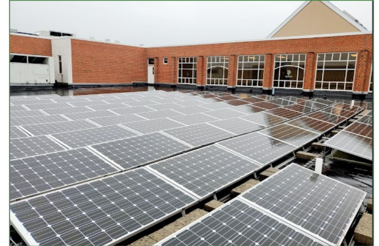
Onsite Renewable Generation System - Solar
